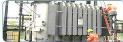
Maintenance of Transformer
